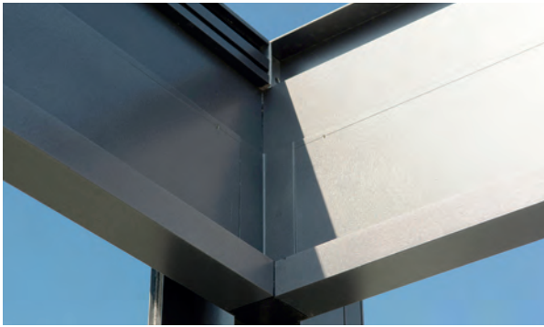
Water run-off in the support
